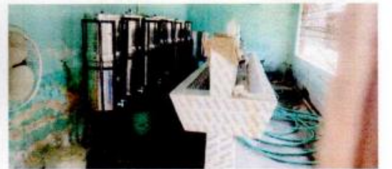
Water filter system in the college
