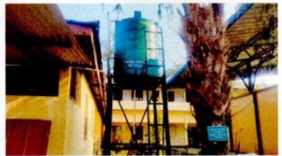
Arsenic treatment plant
